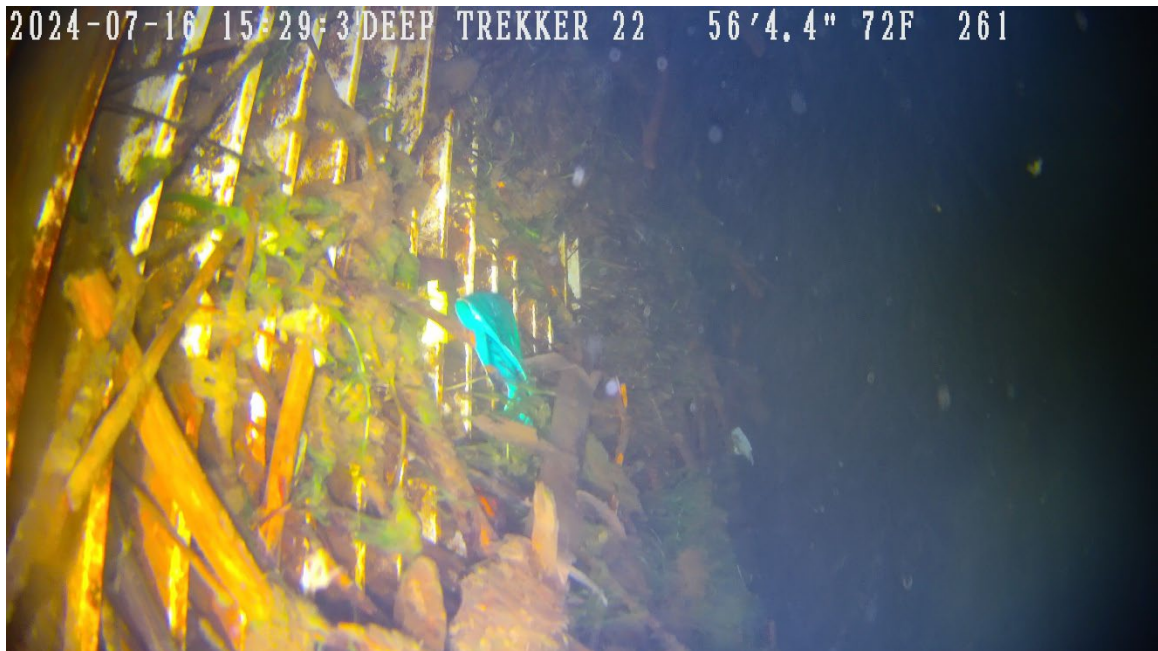
4 Photo: Middle of intake screen After backflush
